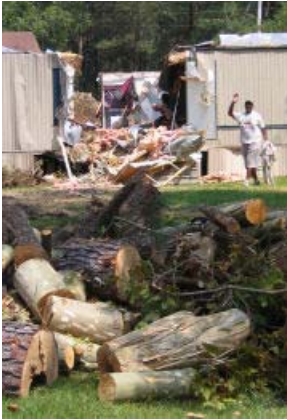
This is John and his house 4 hours after we began the job with all the cut trees piled next to the road where the county will pick them up.
